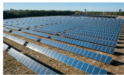
Large, ground-mounted solar (about 1000 kW – or 1 MW - on 5 acres of land, enough to power 100 homes)
