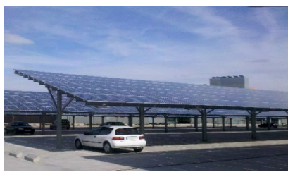
Solar parking canopy (about 100 kW on a half-acre parking lot, enough to power 10 homes)
