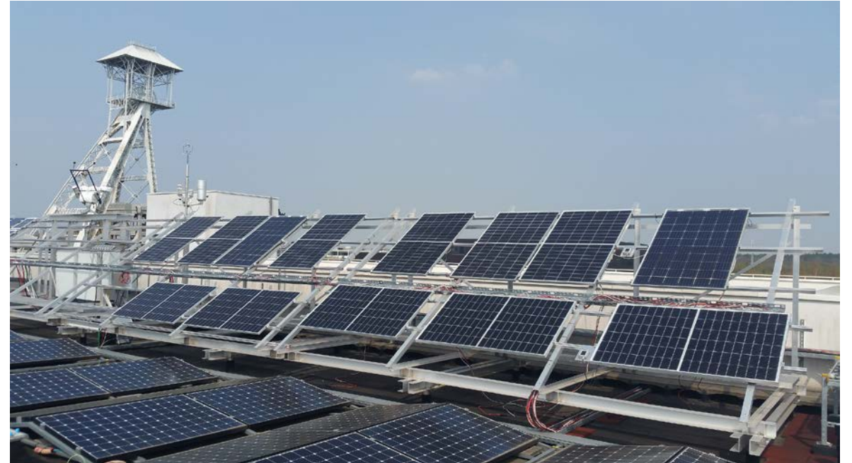
EnergyVille 1 PV test setup [2]
