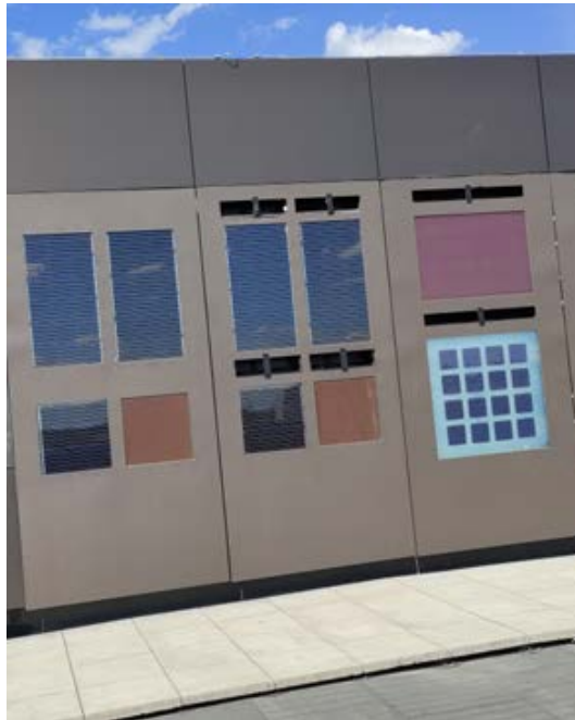
Building integrated PV
