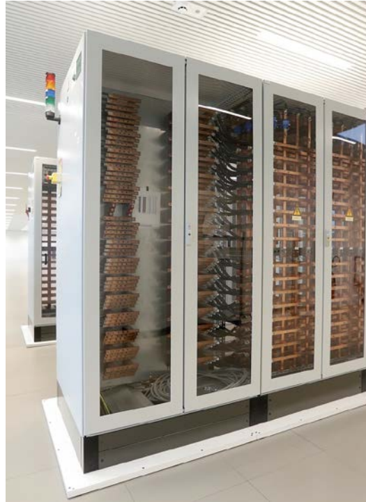
Low Voltage DC
