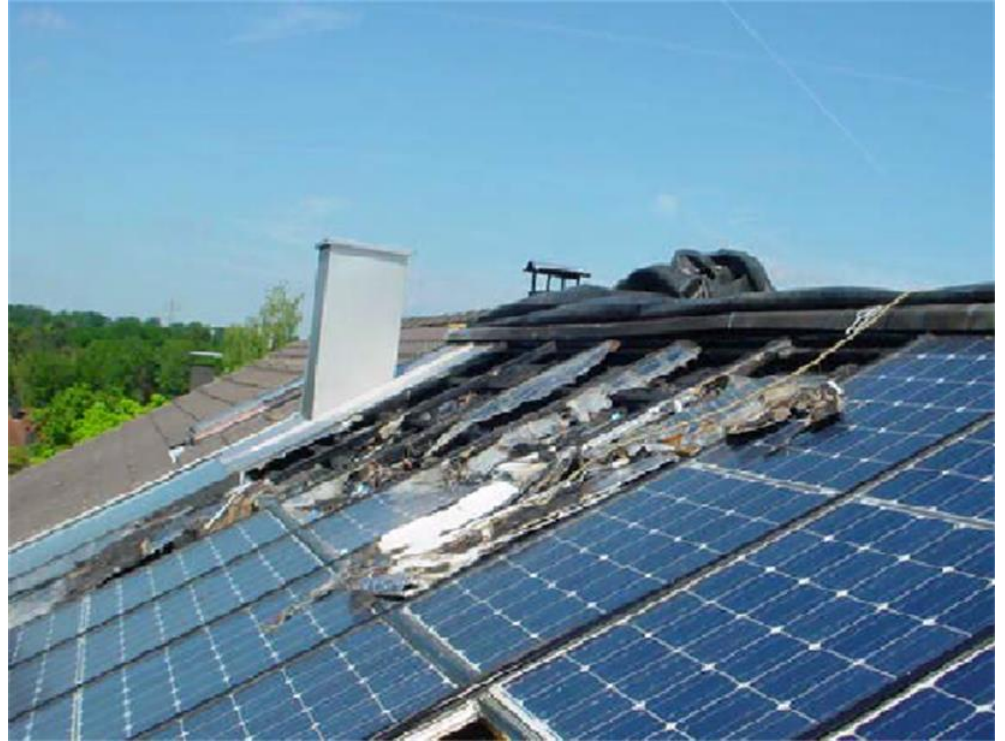
Roof fire caused by ground fault
