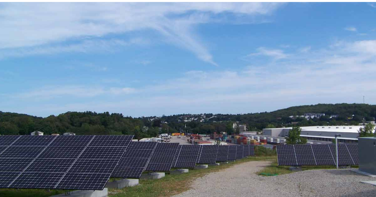
Utility-scale solar photovoltaic plant on capped landfill in Worcester, MA. Photo by Teresa Wheeler, NREL 881278
