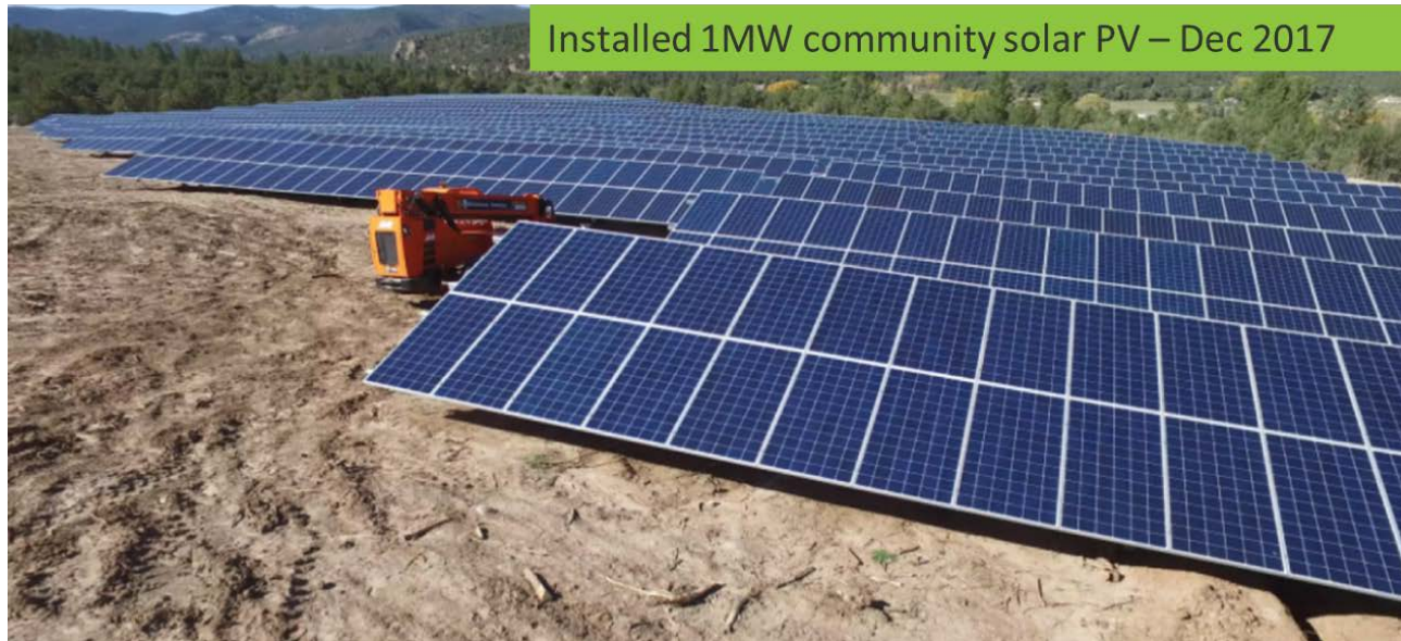
Picuris Pueblo of New Mexico PV Array. 1.0 MW AC , Fixed tilt.
