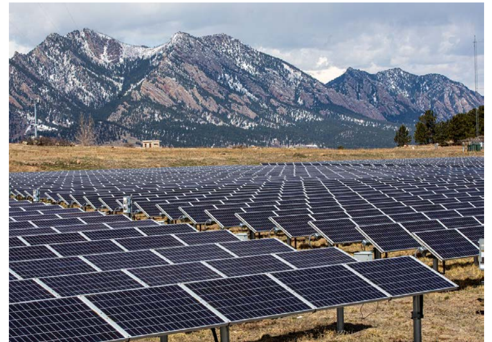
Flatirons Campus PV Array. 1.0 MW AC , One-axis tracking
