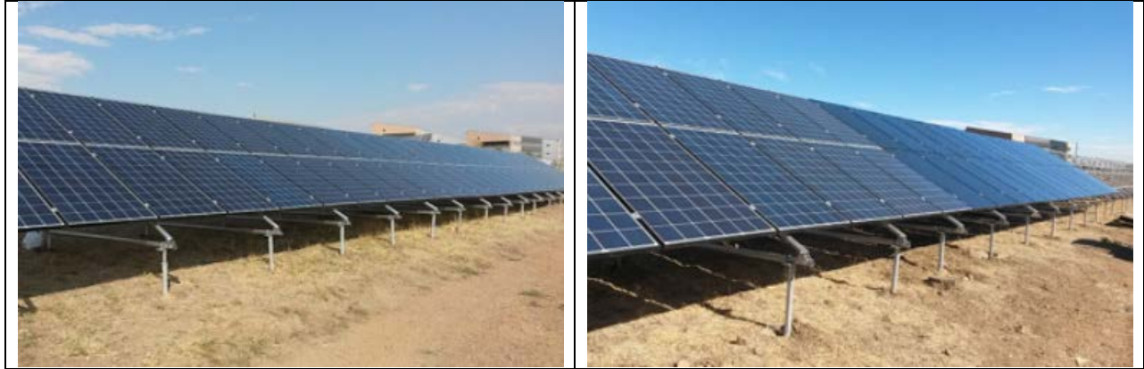
Figure 2. NREL PV Lifetime installations. Jinko Solar (left) and Trina Solar (right)
