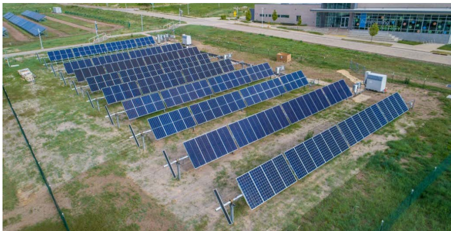
Figure 8. NREL 75-kW tracking PV system supporting PV Lifetime performance data
