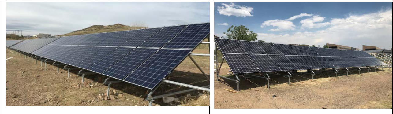
Figure 5. NREL PV Lifetime installations. QCells (left) and Panasonic (right)
