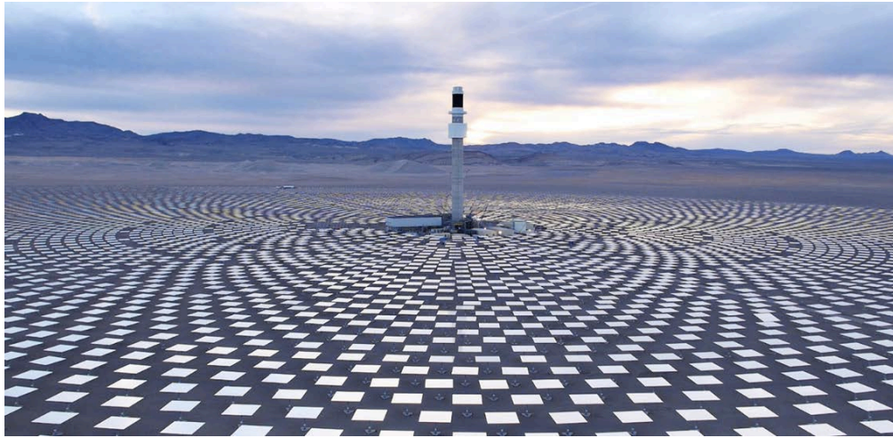
[Crescent Dunes CSP Plant, Tonopah, NV]
