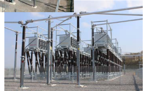
SSSC APFC (3 substations) (UK)
