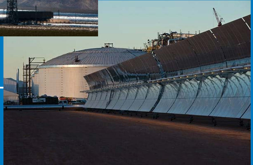
Solana CSP Plant in Arizona, courtesy Abengoa Solar Parabolic trough plant with 6-h storage → too expensive!
