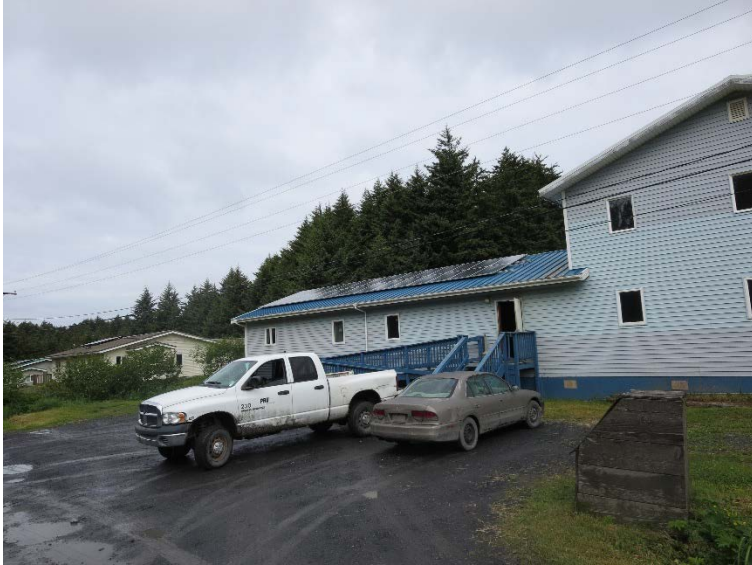
Figure 15. Solar PV array on the Ouzinkie Cultural Center. Photo from Alice Orrell, PNNL.
