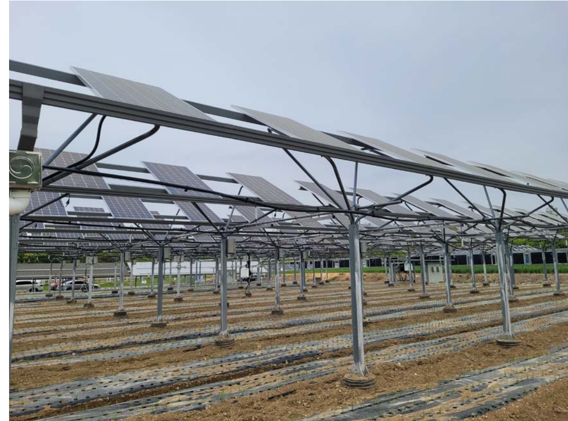
Elevated agrivoltaic system with gutters at Yeungnam University, South Korea (Photo source: Jordan Macknick, NREL)
