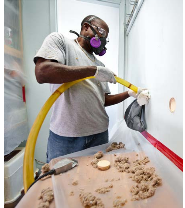
William Stewart with Veterans Green Jobs blows cellulose insulation in the interior walls of this Lakewood, Colorado, home. Photo by Dennis Schroeder, NREL 17964
