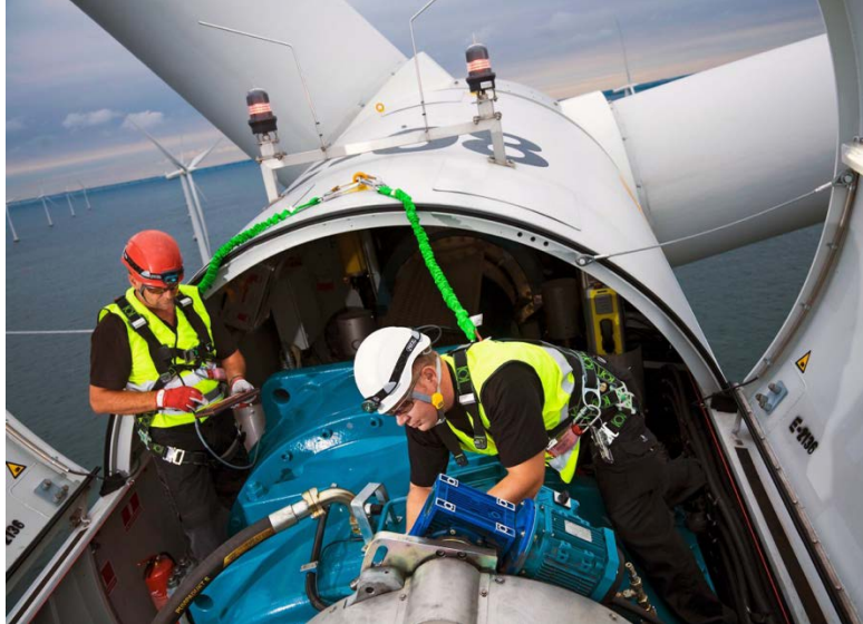
Figure 51. Engineers work in the nacelle of an offshore wind turbine at the Lillgrund Offshore Wind Farm in Sweden in 2008. Photo from Siemens AG
