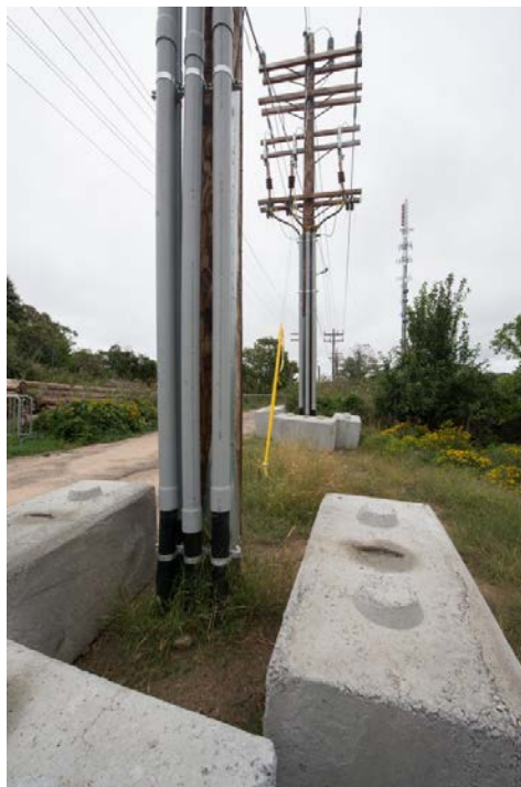
Figure 24. Upgraded grid infrastructure on Block Island, Rhode Island, after the construction of the Block Island Wind Farm. Photo from Dennis Schroeder, NREL 40394
