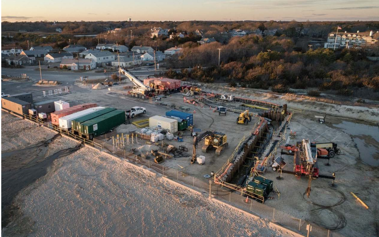
Figure 25. Construction occurs in the parking lot at Covell's Beach in Barnstable, Massachusetts, the location where cables from the Vineyard Wind 1 project come onshore. Following the completion of construction, this trench was covered, leaving no lasting visual impact or impact on use of the area. Photo from Robin Lubbock, WBUR
