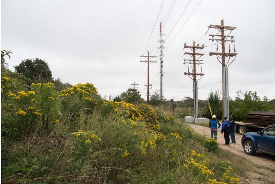
Figure 28. Transmission infrastructure on Block Island, Rhode Island. The island saw transmission infrastructure upgrades as part of the Block Island Wind Farm project. Photo from Dennis Schroeder, NREL 40487
