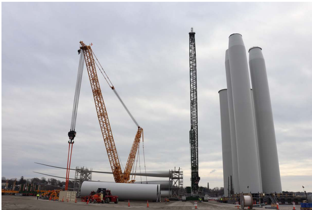
Figure 8. Tower components for the South Fork Wind project await transportation at State Pier in New London, Connecticut. Photo from Matilda Kreider, NREL
