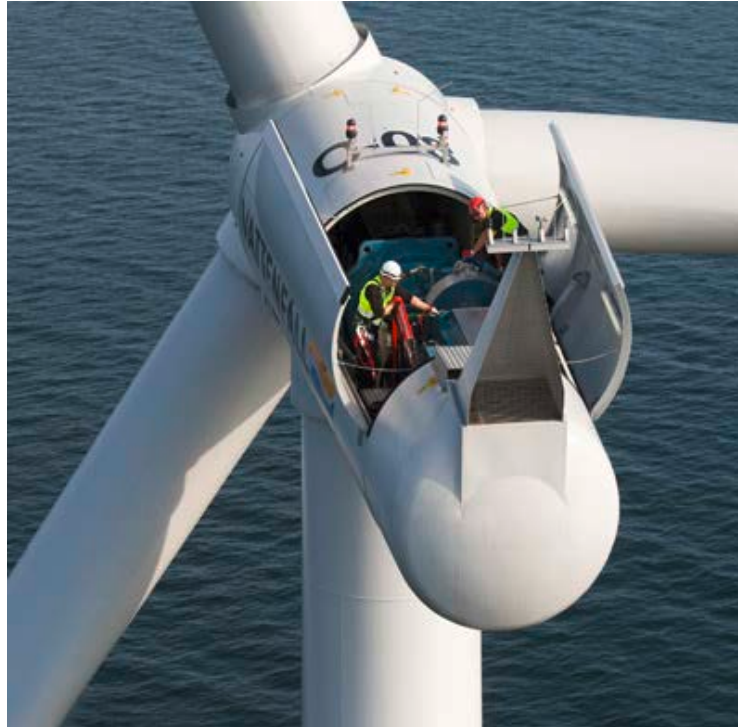
Figure 49. Maintenance is performed on a turbine at the Lillgrund Offshore Wind Farm off the coast of Sweden. Photo from Siemens AG 27853
