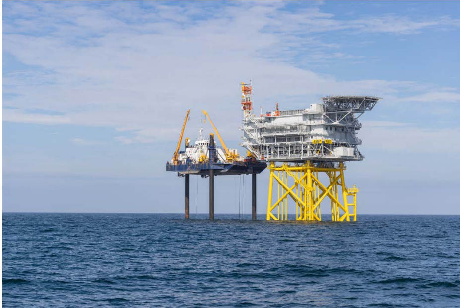
Figure 15. An offshore substation under construction in the Vineyard Wind 1 project off of Massachusetts. Photo by Joe DeINero, NREL 90966
