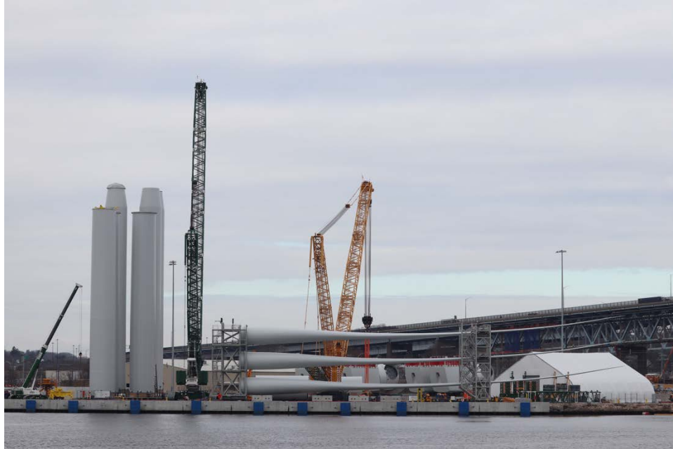
Figure 45. Components for the South Fork Wind project sit at State Pier, an offshore wind marshaling terminal in New London, Connecticut, awaiting transportation to the project site off of Long Island, New York. Photo from Matilda Kreider, NREL
