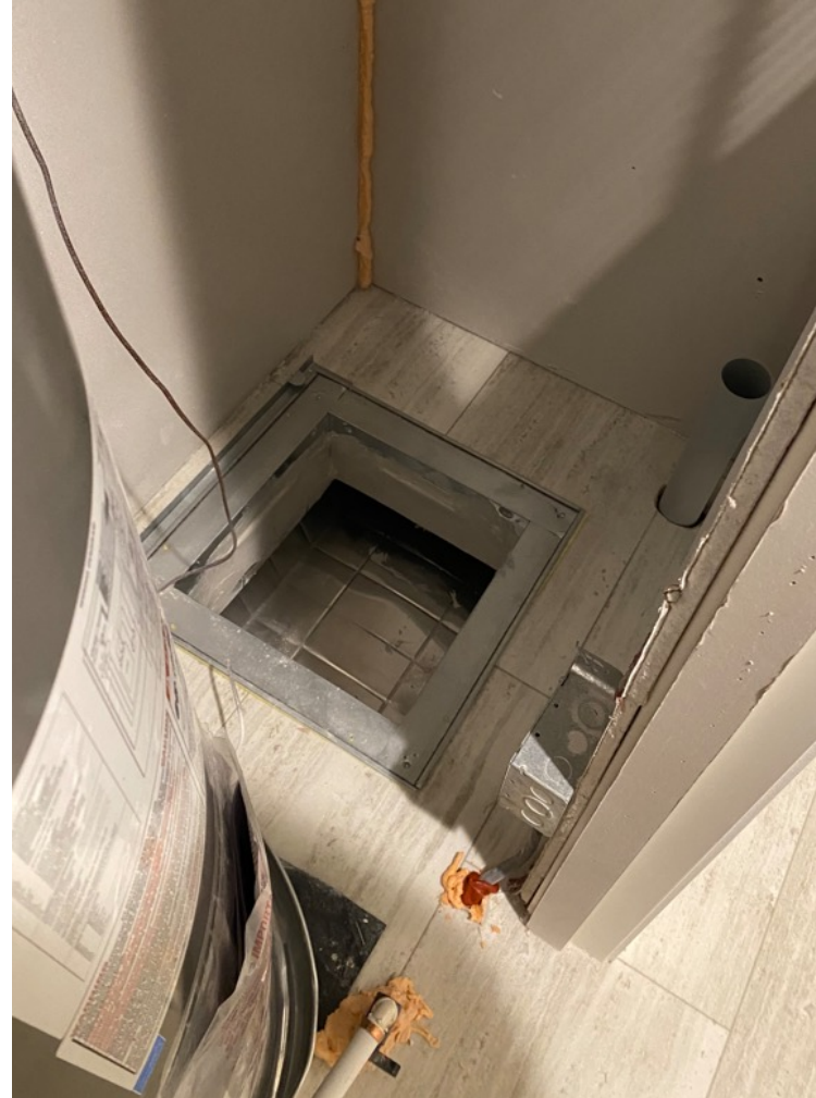
Heat pump ready with sealed plenum, conduit for refrigerant lines, thermostat wiring, and wiring for backup strip heater. Photo from Peter Schneider, VEIC
