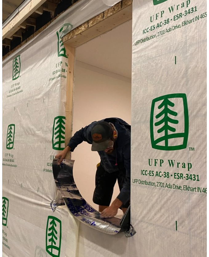
Integrating house wrap and window flashing prior to window installation. Photo from Peter Schneider, VEIC.
