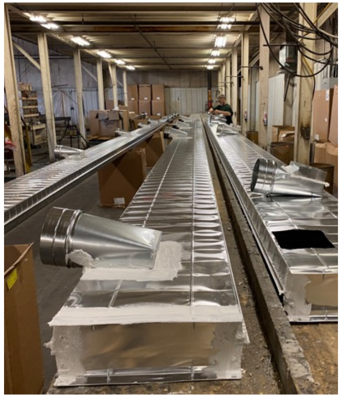
Fabricating duct system off assembly line and duct sealing with mastic. Photo from Peter Schneider, VEIC.
