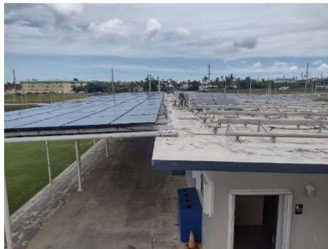
Figure A-6. Array on northeast roof (right) suffered much more damage. Racking was higher off the roof.
