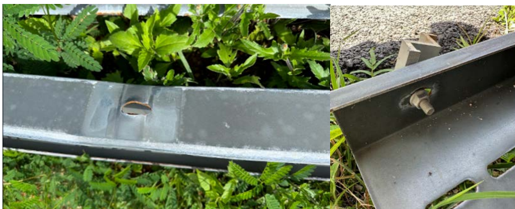
Figure 32. Evidence of direct bolt tear-out of racking rails (left) and steel deformation from a top-clamp bolt that was close to tearing out (right)
