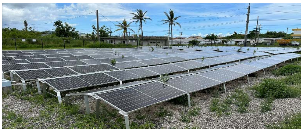
Figure 69. Upon close inspection, modules in this array are deformed and sagging. While it did not suffer any obvious damage from the typhoon, this will likely impact production and leaves the array more vulnerable to damage from future events.
