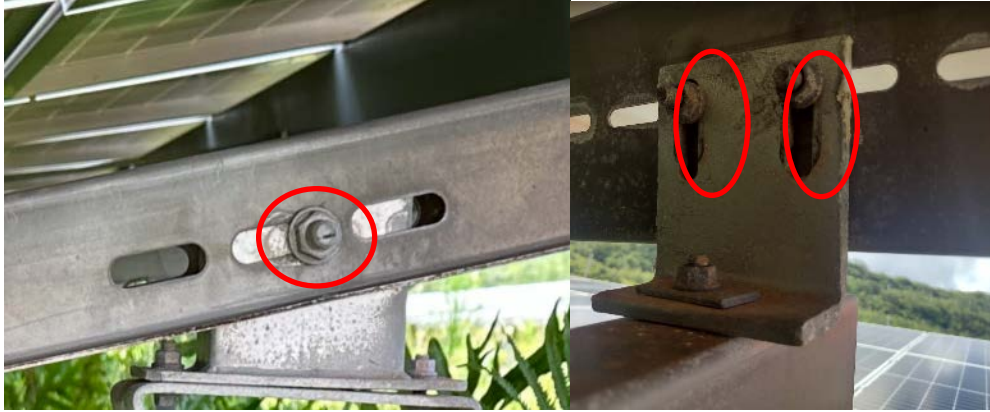
Figure 47. Racking bolts that slipped in slotted connections, clearly shown by impressions left from the original position of the bolt. Bolts may have loosened due to wind-induced vibrations and then slipped.
