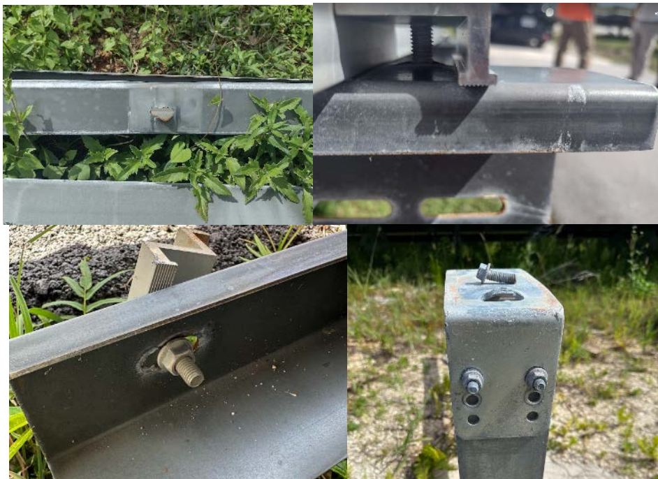
Figure 48. Various instances of bolt tear-out or near tear-out at various places within the racking system
