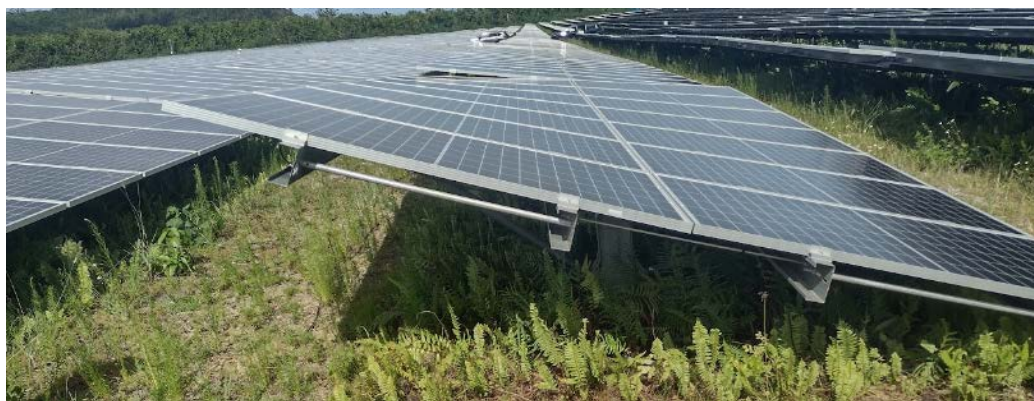
Figure 70. Racking deformation or shifting has led to some modules raised higher than others. These sections of the array are likely more exposed and racking components are more fatigued, leaving it more vulnerable to damage from future wind events.
