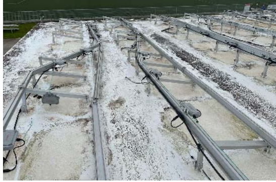
Figure 51. Roof corner zones, especially on roofs without parapets, experience the highest wind loads and often experience the most damage (as shown here)
