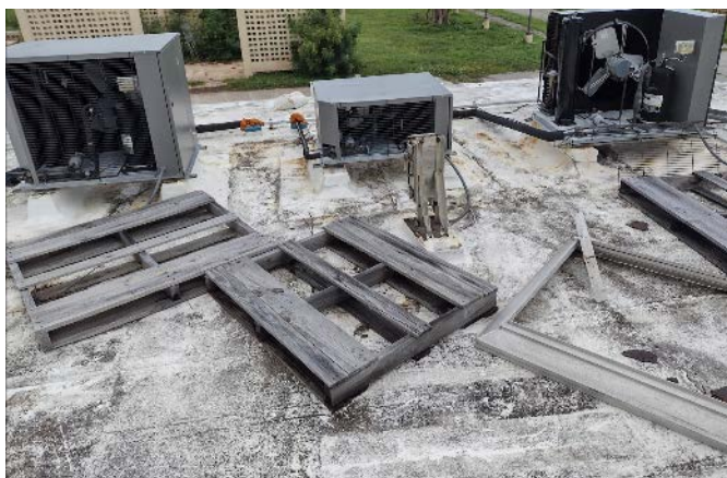
Figure 67. Debris left on rooftop after the typhoon
