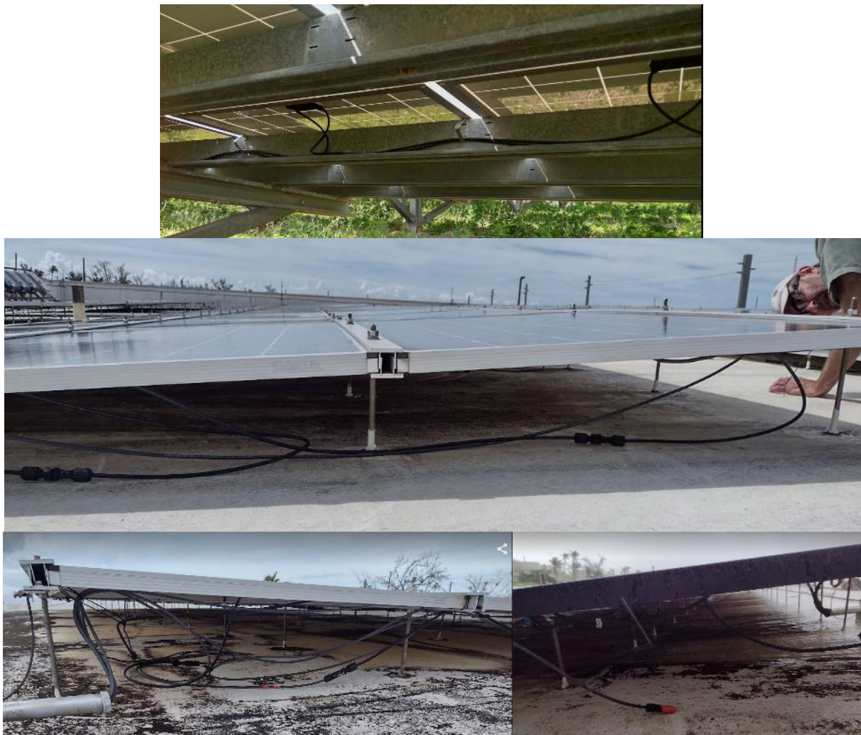
Figure 53. Various wire management approaches—some good, some bad—and failures. Top: Metal PV-specific wire management system that has held wires in place for more than 10 years. Middle: Wires and PV connectors down on the roof are a safety and fire risk due to potential water damage and insulation damage as wind drags them across the roof surface. These were likely tied under the panels with plastic or nylon wire ties that failed. Bottom left: More wires and connectors down on roof surface, likely because of failed wire ties. Notice the one plastic wire tie under the left side of the module. Bottom right: A PV connector that has come unattached, breaking the circuit and stopping power delivery from a whole string of PV modules.
