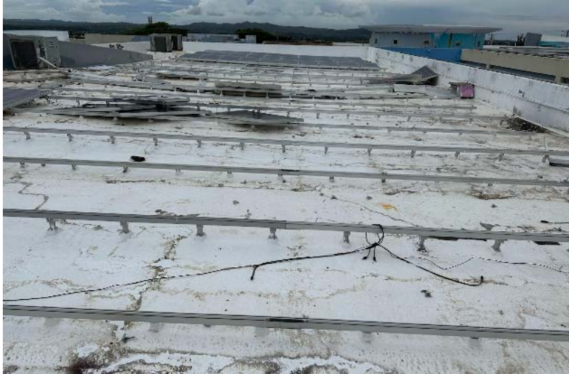
Figure 10. Catastrophic failure: modules blown of racking at Guam Community College. This is most likely not a module failure, but a failure of the module attachments.
