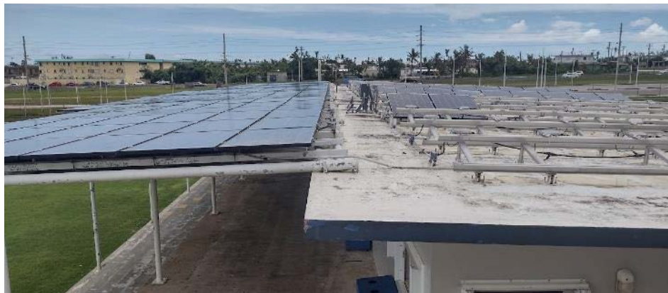
Figure 42. The right section of this array had a high tilt angle (14°) and suffered extensive damage. The left portion of the array was mounted flush to the roof at a low tilt angle (4°) and suffered no damage.
