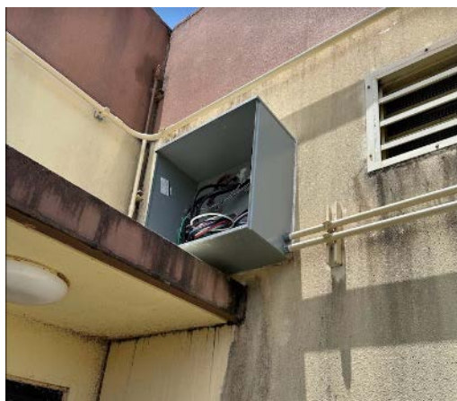
Figure 56. Electrical pull box with missing cover, likely blown off during the storm. The box does not appear to be rated for the conditions; it is likely a NEMA 3-rated enclosure. This leaves the system vulnerable to water ingress that could flow through the conduit into other electrical components such as inverters and AC breaker panels.
