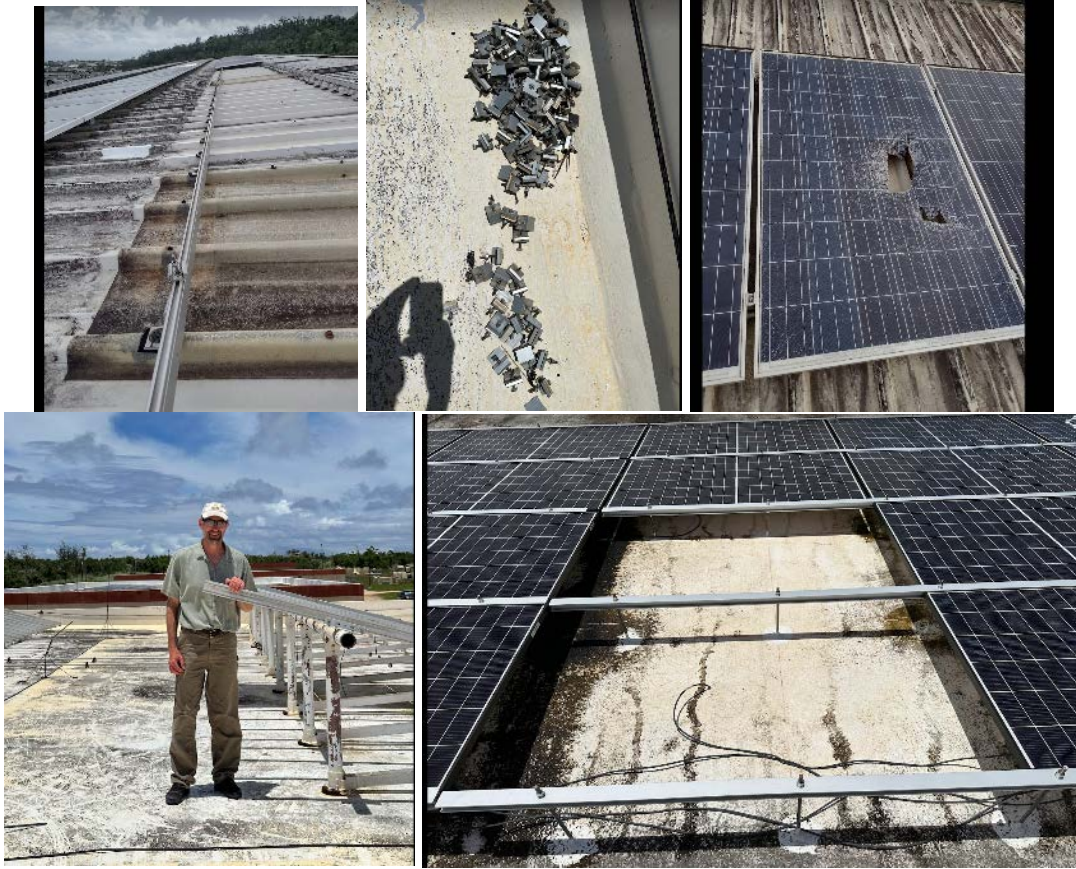
Figure ES-1. The most common failure modes, clockwise from top left: (a) Inadequate clamping of module frame to mount, leading to cascading failure. Module mounting clamps in this case rotated out of the support rail and can be seen on the roof in (b). (b) Undamaged module clamps remaining on roof surface after they rotated out of the racking and released modules. (c) Module damage from debris impact. (d) Modules that released from the mounting system. (e) System with excessive tilt angle.
