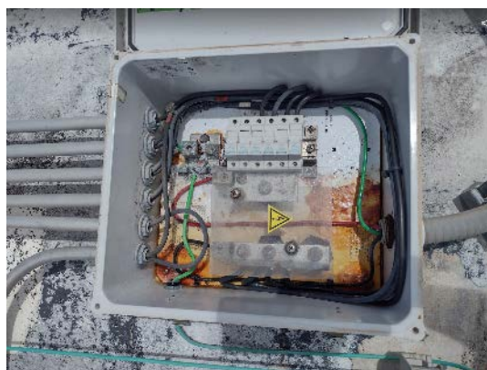
Figure 54. Combiner box damaged from water intrusion. This box was NEMA 4X rated, but still not of high enough quality.
