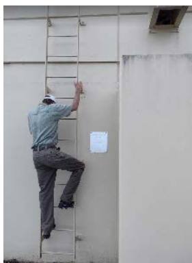
Figure 63. An example of good rooftop and PV array access from an outside ladder. Some buildings did not have easy roof access, impeding maintenance and damage assessment.
