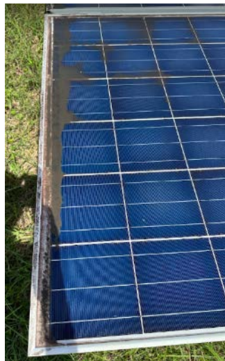
Figure 60. Algae buildup along the frame on the lower side of PV modules. This site is experimenting with algaecide to mitigate buildup.
