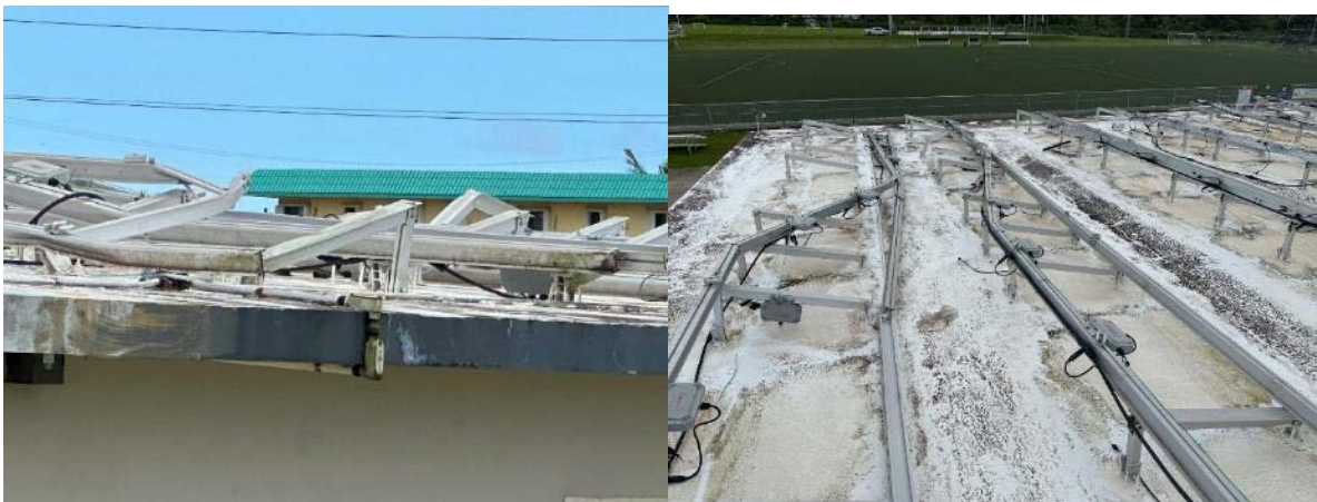
Figure A-5. Racking destroyed near roof corner that likely experienced the highest wind loads
