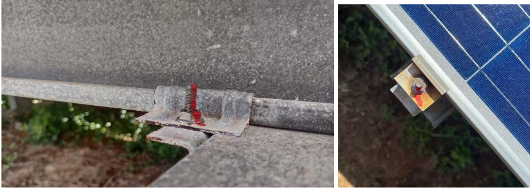
Figure 39. Torque stripes on torqued bolts can give a visual indication if bolts have loosened over time. The bolt on the left is in line. The bolt on the right appears to have rotated loose slightly.
