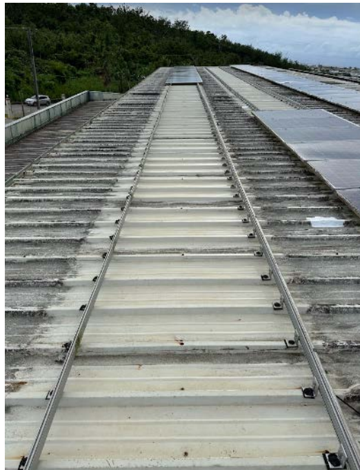
Figure 20. Cascading/progressive failure of two rows of modules that were held with top clamps. One (or a small number) of failures can lead to the loss of many neighboring modules. This is because the top clamps used require the presence of two adjacent modules to maintain adequate clamping force. If one module comes loose, the whole row is vulnerable to failure.
