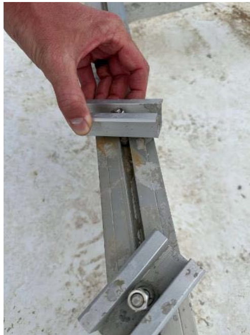
Figure A-8. Module clamps appeared to have loosened. Split washers do not provide locking capability.
