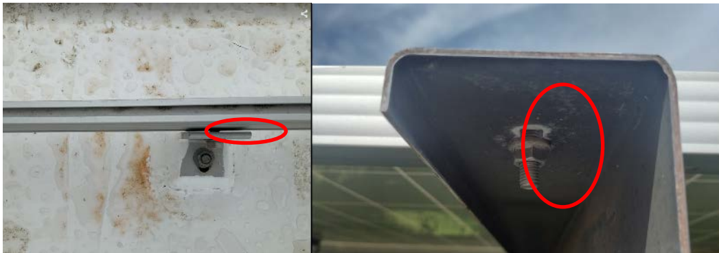
Figure 46. Left: Loose bolted connection between roof anchor and racking rail. Bolts were loose down the entire length of this rail, and it could move easily. Right: A loose nut on a bolted connection.
