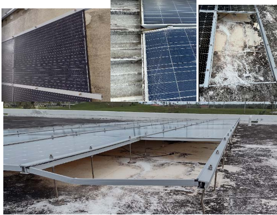
Figure 13. Module damage with undetermined cause, only seen on five of the hundreds of thousands of panels seen on the trip. Top left: Cracked glass with no clear impact point; top middle: module frame bent; top right and bottom: module frame remaining in racking with the rest of the module missing.
