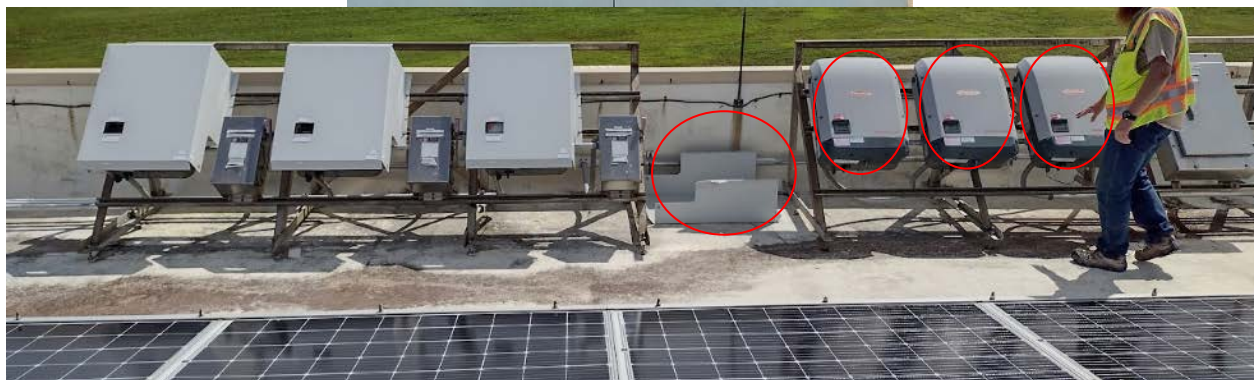
Figure 58. Shade covers blown off inverters; low-impact and low-priority failure. Notice the faded labels on the disconnect boxes, too.
