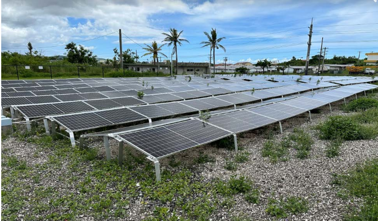
Figure 44. The lack of a substantial racking system on this “east-west” ground-mounted system puts extra loading onto the modules themselves. Modules in this array are deformed, sagging in the middle. They are vulnerable to damage in a future event and could have suffered internal damage that might diminish power production or shorten useful life.
