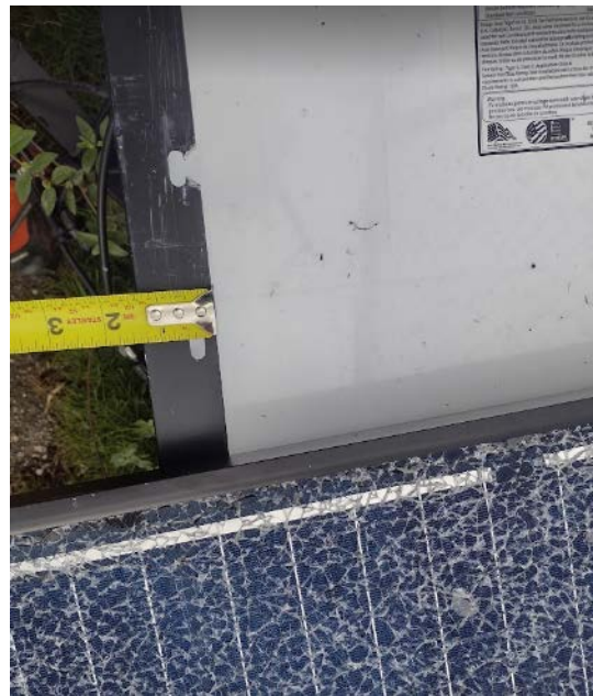
Figure 66. The predrilled bolt slots on this module were very close to the edge of the module frame lip, allowing the bolts to tear out of the frame more easily. Larger-diameter washers could help.
