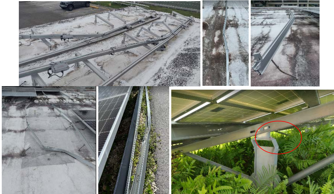
Figure 40. Deformation of various racking components. Top left experienced higher loads due to its location near the roof corner. Top middle, top right, and bottom left used too thin gauges and low-quality components. Bottom middle and bottom right were likely the result of extreme loads and bolts that slipped in their slotted connections.
