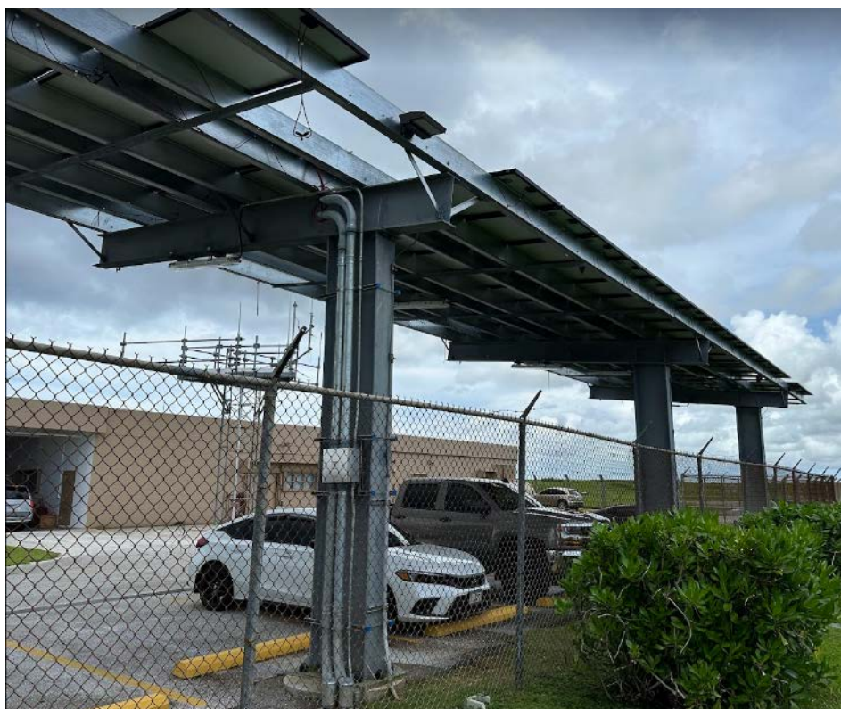
Figure 65. PV carport structure with isolated missing modules where modules tore off the bolts holding them down. The structure is also very tall (approximately 20 feet high) and thus susceptible to higher wind loads.
