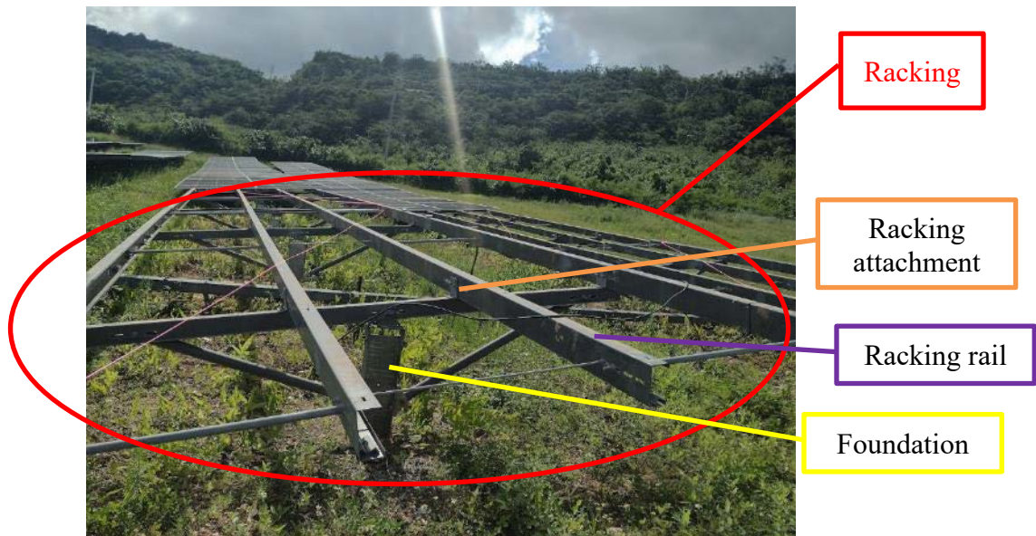
Figure 5. A PV racking system onto which modules are mounted.
