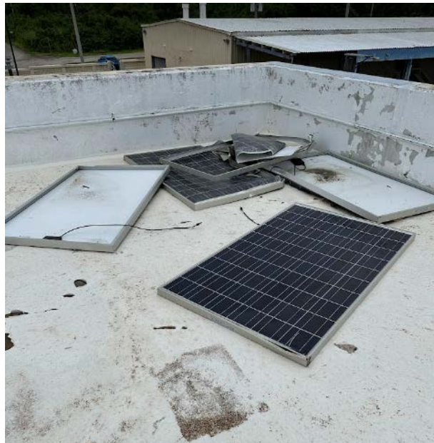
Figure 11. Damaged modules that came free of racking scattered around a rooftop. It often cannot be determined if modules were damaged before or after coming free.
