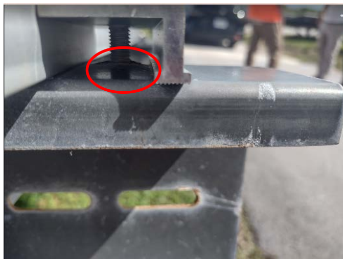
Figure 33. Steel deformation where a bolted joint was likely overtightened during installation
