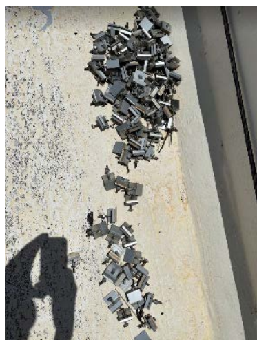
Figure 25. Unirac Pro Series T-bolt clamps that rotated free of the racking littering a rooftop. Note that clamps do not show signs of deformation or damage, implying they came free from the racking relatively easily.
