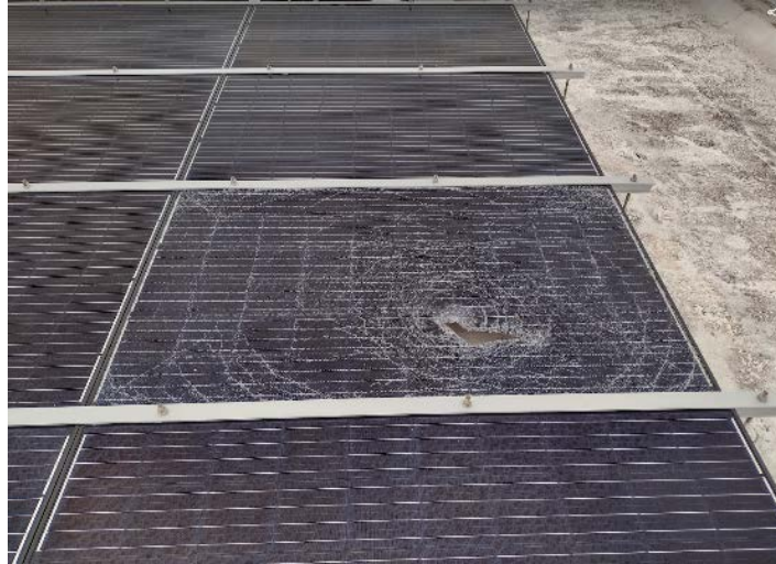
Figure 12. Module intact in racking damaged from flying debris
