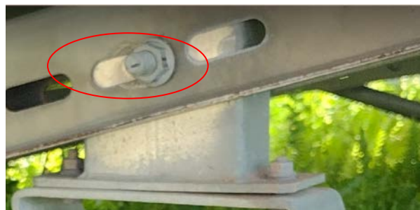
Figure 49. Clamp separation between two racking members. This could be a secondary failure as a result of other racking system failures that allowed movement in the racking system.
