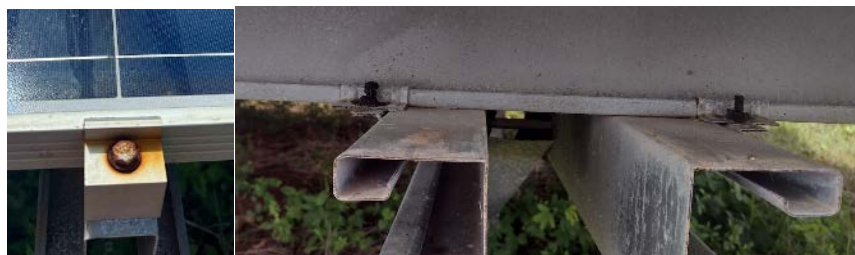
Figure 62. Salt mist and humidity make Guam a very corrosive environment (rated C5 on the International Organization for Standardization’s (ISO) corrosivity scale). This can cause signs of corrosion where dissimilar metals contact. We saw corrosion on infrastructure attachments on Guam. It was typically worse on non-PV infrastructure. We saw no failures related to corrosion.
