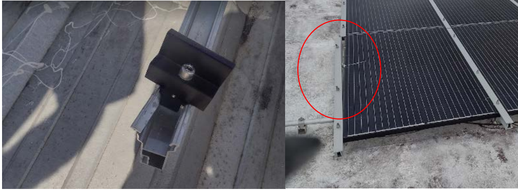
Figure 43. Debris impact can damage racking, which may free modules
