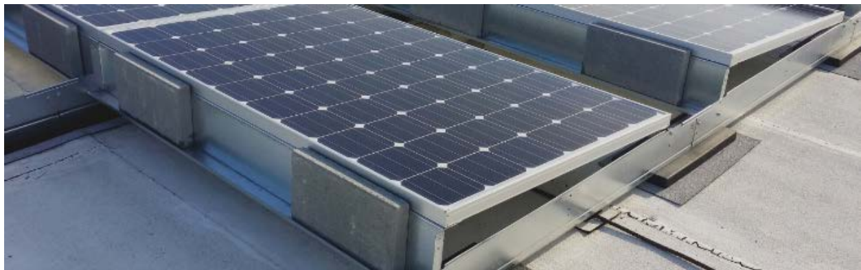
Figure 52. Rooftop solar system with wind deflectors on rear side to block wind and prevent uplift forces
