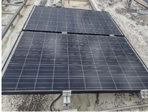
Figure 36. Clamps should be installed on modules as required in installation manuals, not off-center as shown here
