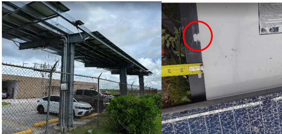
Figure 34. One carport system on Guam lost modules due to bolts tearing out of the module frames and due to flying debris. This tall structure mounted the modules about 22 feet above the ground. The modules had two potential bolt slots; only one was used. These slots were also close to the edge of the module frame where the bolts tore through (right).
