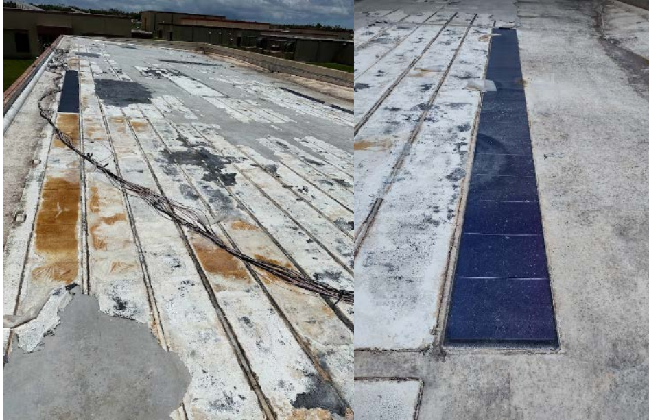
Figure 45. One system that used an adhesive to attach solar directly to the roof surface was nearly totally blown away. Although this product is no longer on the market, avoid systems like this that use adhesives or attach solar directly to the roof.
