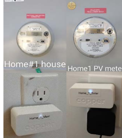
Utility meters and Copper gateway
