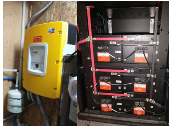
SMA Sunny Island battery inverter
