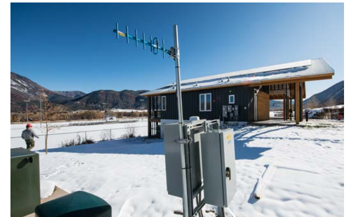
Communication box and service transformer
