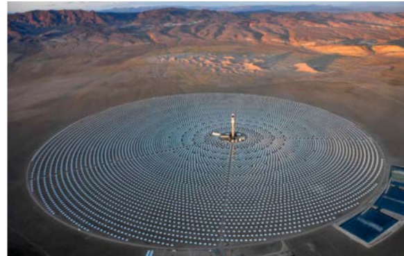
110-MWe Crescent Dunes Solar Plant with 10-hour Thermal Energy Storage
