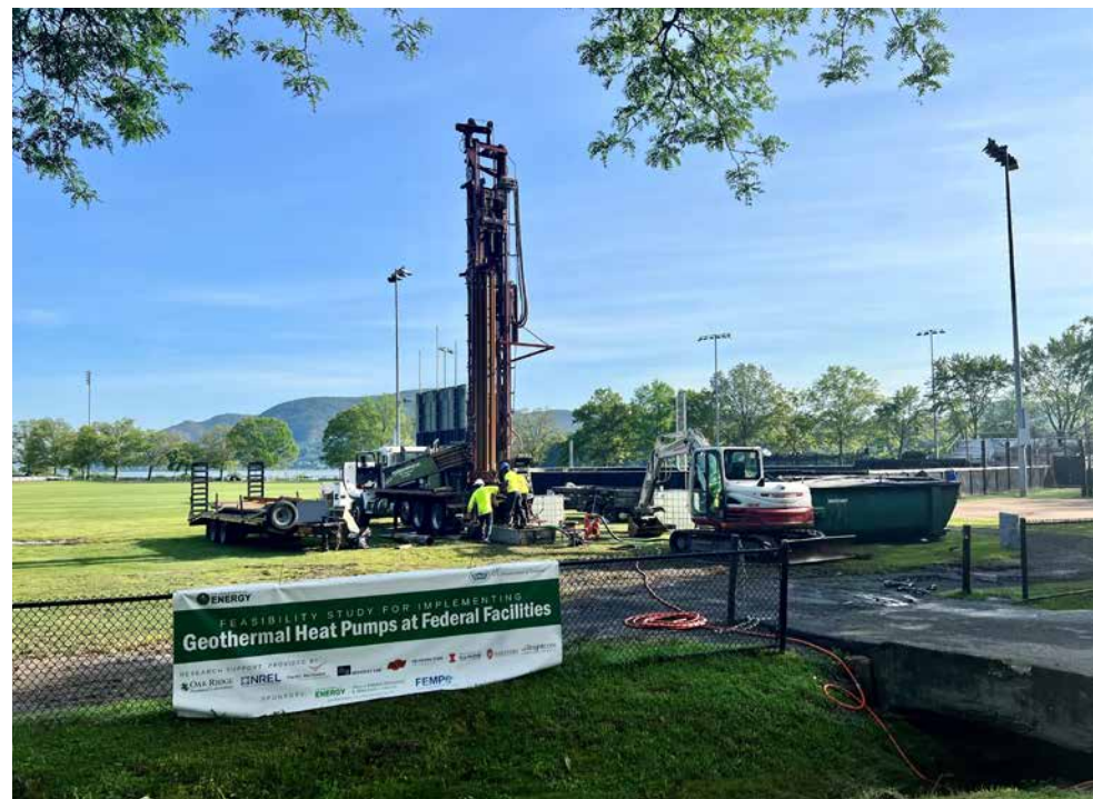
Well drilling for tests characterizing geo exchange resource potential at the West Point North Athletic Field Complex. Photo courtesy of Bass Shakra, Energy Manager, DPW, West Point
