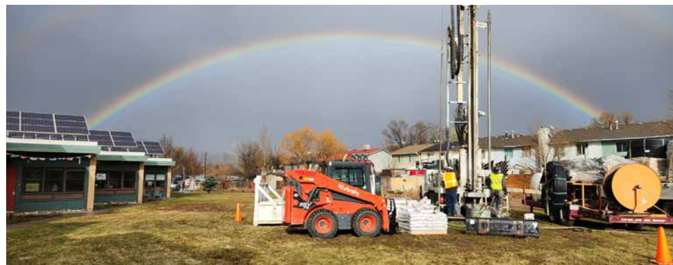
The Carbondale Community Geothermal Coalition is focused on enabling a zero energy district in Carbondale, Colorado. Photo from Aaron Orelup, GreyEdge Group
