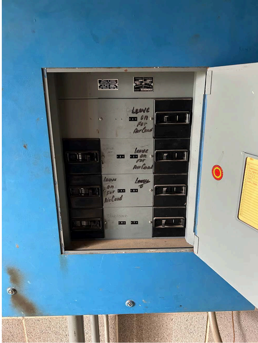
Figure 10. SOD-A 240-V/416-Y blue service panel
