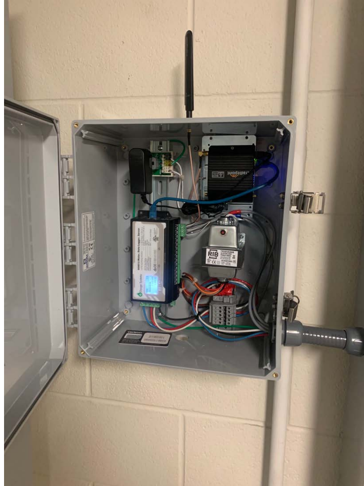
Figure 4. Metering system installed at B8 JOC at Camp Mabry
