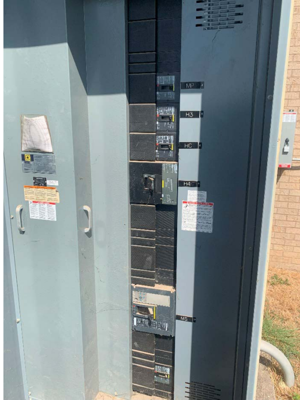
Figure 5. Camp Mabry SCIF dedicated service panels
