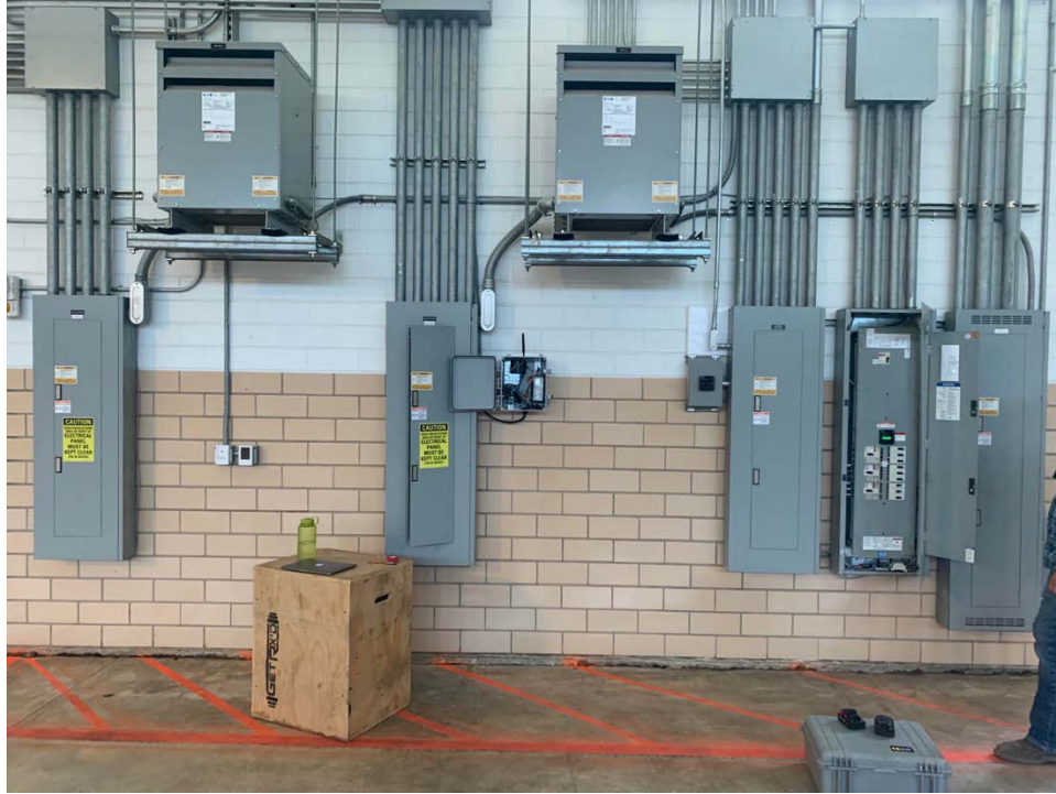
Figure 12. San Marcos RC service panels with metering installed at center (right to left: MDP, HA, EMHA, EMLA, LA).
