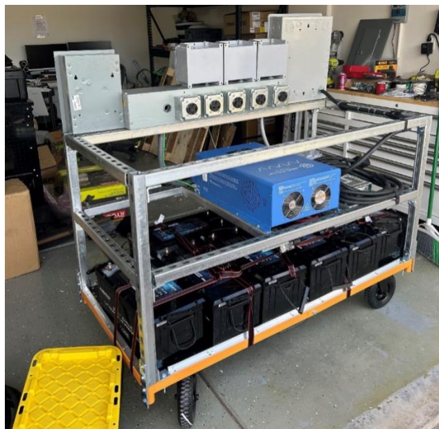
Figure 3. B&B Technology Solutions' skid from the back
