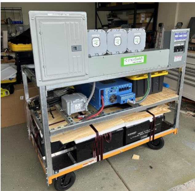
Figure 2. B&B Technology Solutions' skid from front
