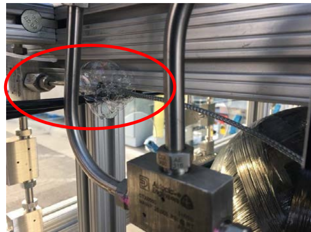
Small leak identified by a soap solution
