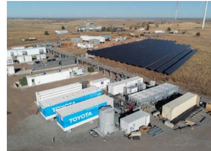
The ARIES facility Large scale H 2 production and power generation; available for H 2 release studies (commissioned in January 2024).
