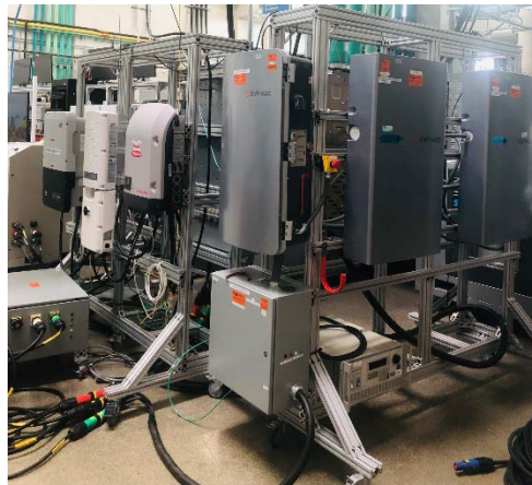
Section 2 (single-phase): 15 kVA GFM 3, 15 kVA GFL)
