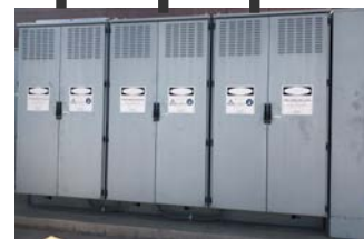
Load bank (1 MW)
