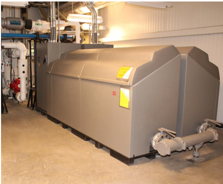
Figure 12 - Hydraulic Power Units
