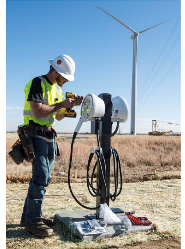
Installation of smart charging system at NREL's Flatirons Campus (Dennis Schroeder / NREL )
