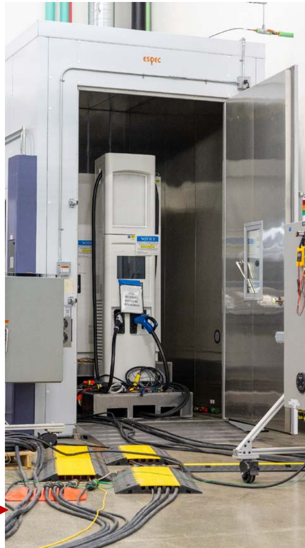
EVSE and Power Cabinets in Thermal Chamber
