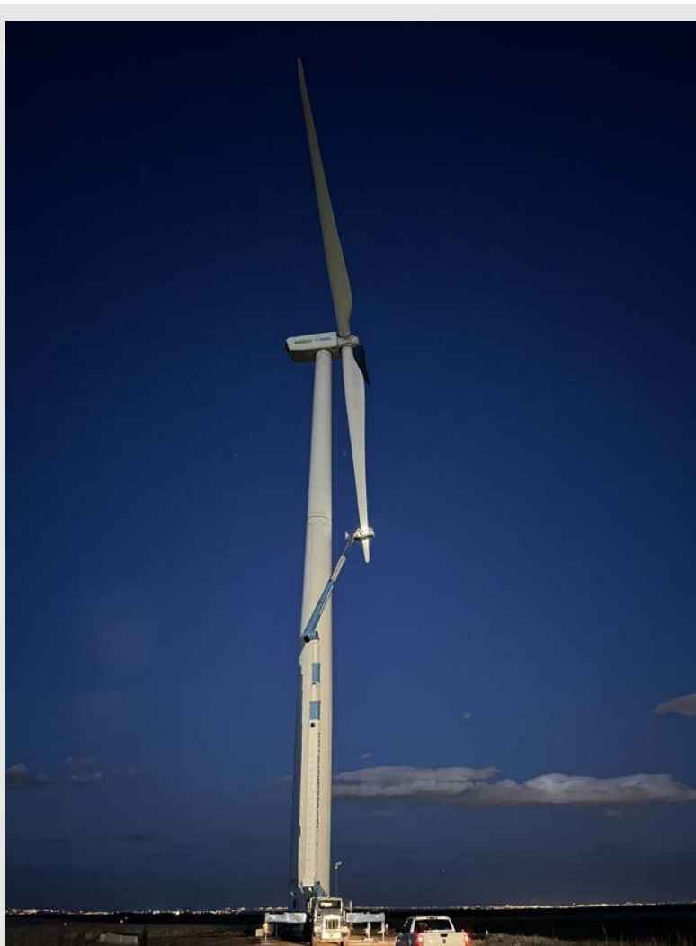
Evening work on the GE 1.5-MW wind turbine located at NREL Flatirons Campus. In this photo the team of technicians is removing the DTU pressure belts from one of the three blades after the experiment was successfully completed. Photo by Pietro Bortolotti
