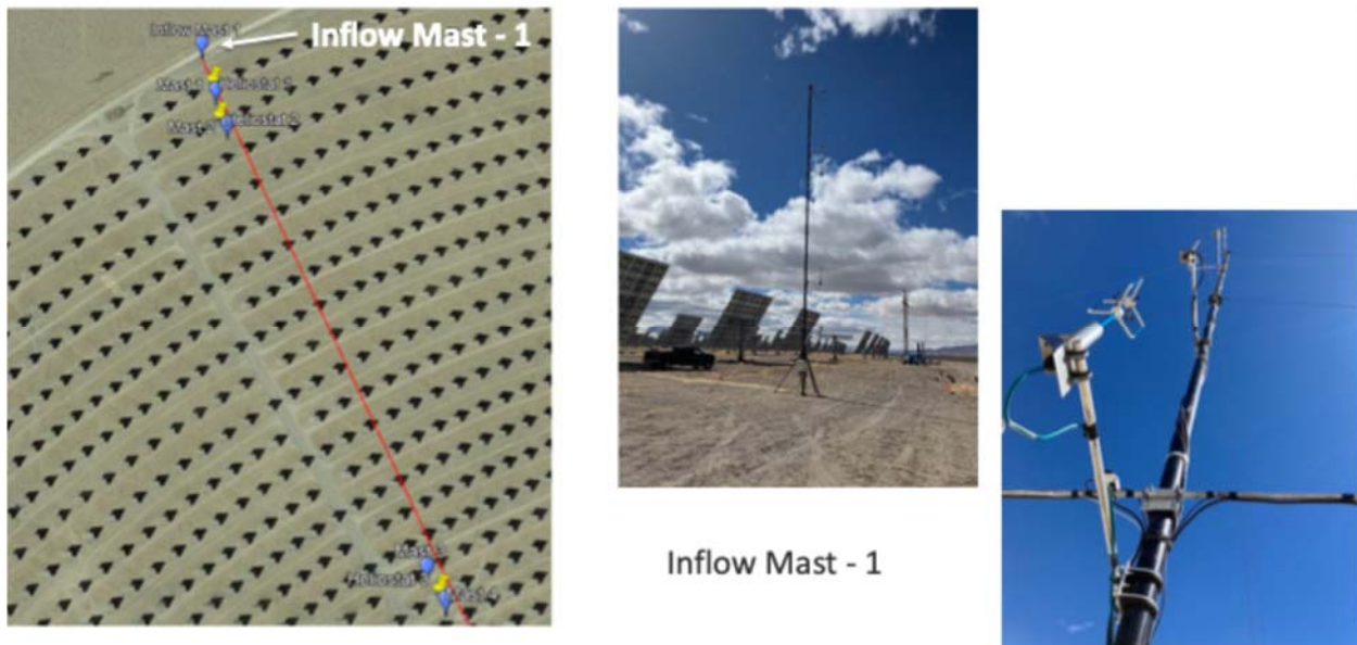
Figure 16: Inflow mast installed at Crescent Dunes power plant.
