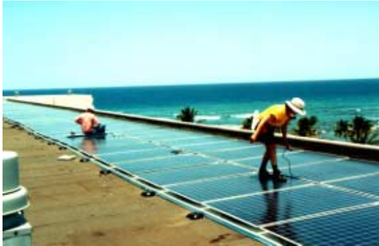
Figure 3. New array performance characterization methods were applied to a roof-integrated PowerLight system with 100-kW array of modules from ASE Americas.
