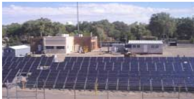
Figure 1. Sandia National Laboratories' Inverter Test Facility
