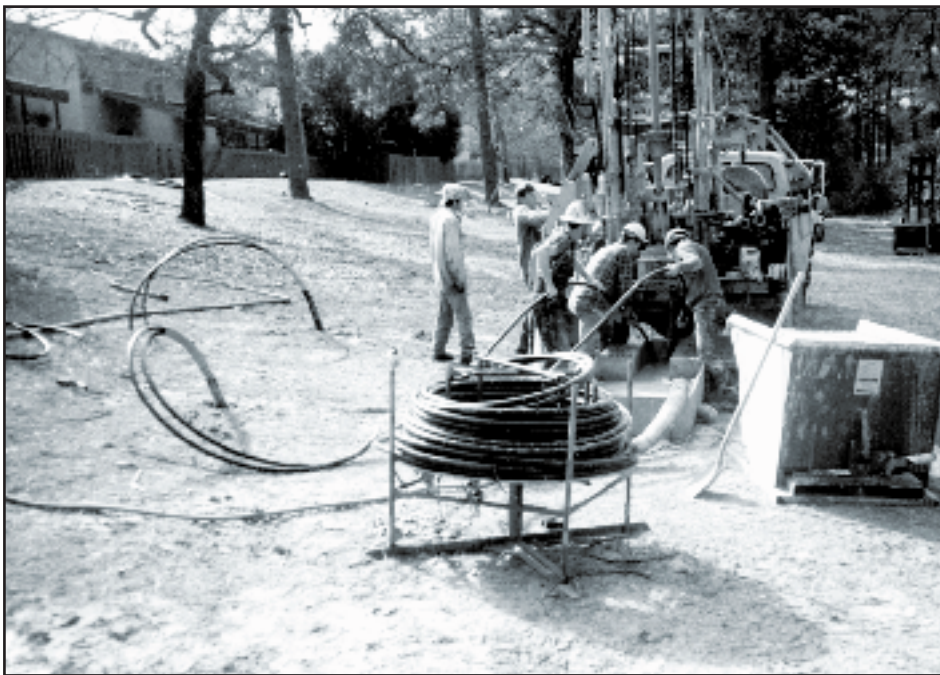
Installation of a geothermal heat pump requires drilling two boreholes which are 4 inches in diameter and range from 125 to 450 feet deep.
