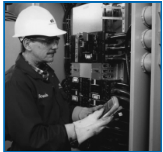
Motor load measurements quantify energy savings.
