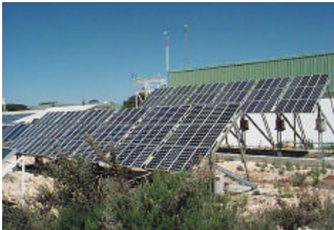
7.5 kW PV field (left)
