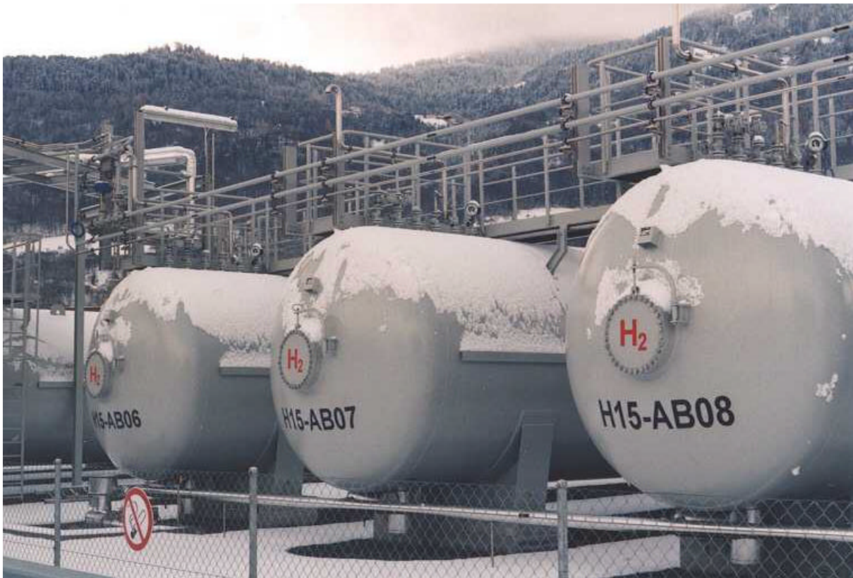
Hydrogen storage tanks at the sapphire production plant of Djévahirdijan SA, Monthey
