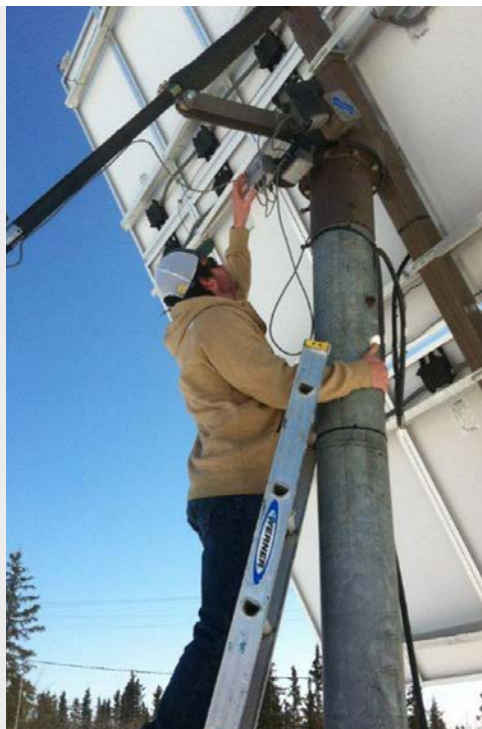
The National Renewable Energy Laboratory's Alex Dane helps repair the tracking motor of a community-owned solar photovoltaic array in Venetie, Alaska, as part of DOE Office of Indian Energy's Strategic Technical Assistance Response Team (START) Program.
