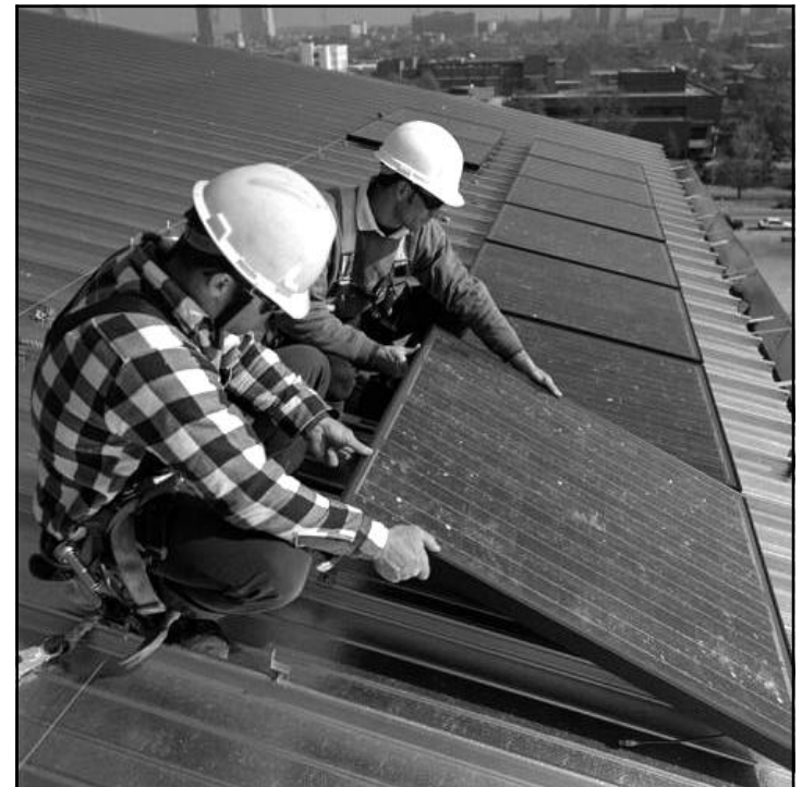
Photovoltaic modules being installed on the roof of the covered swimming pool used for the 1996 Summer Games in Atlanta, Georgia. This 311-kW p , polycrystalline silicon system from Solarex Corporation and Solar Design Associates is connected to the utility grid.
