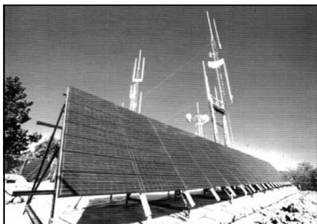
Stand-alone photovoltaic systems provide power to telecommunications equipment such as this in remote locations all over the world.
