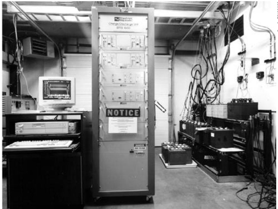
Battery tests sponsored by the PV Program at Sandia Laboratories helped define appropriate charge and set points and predict battery maintenance intervals in PV systems.
