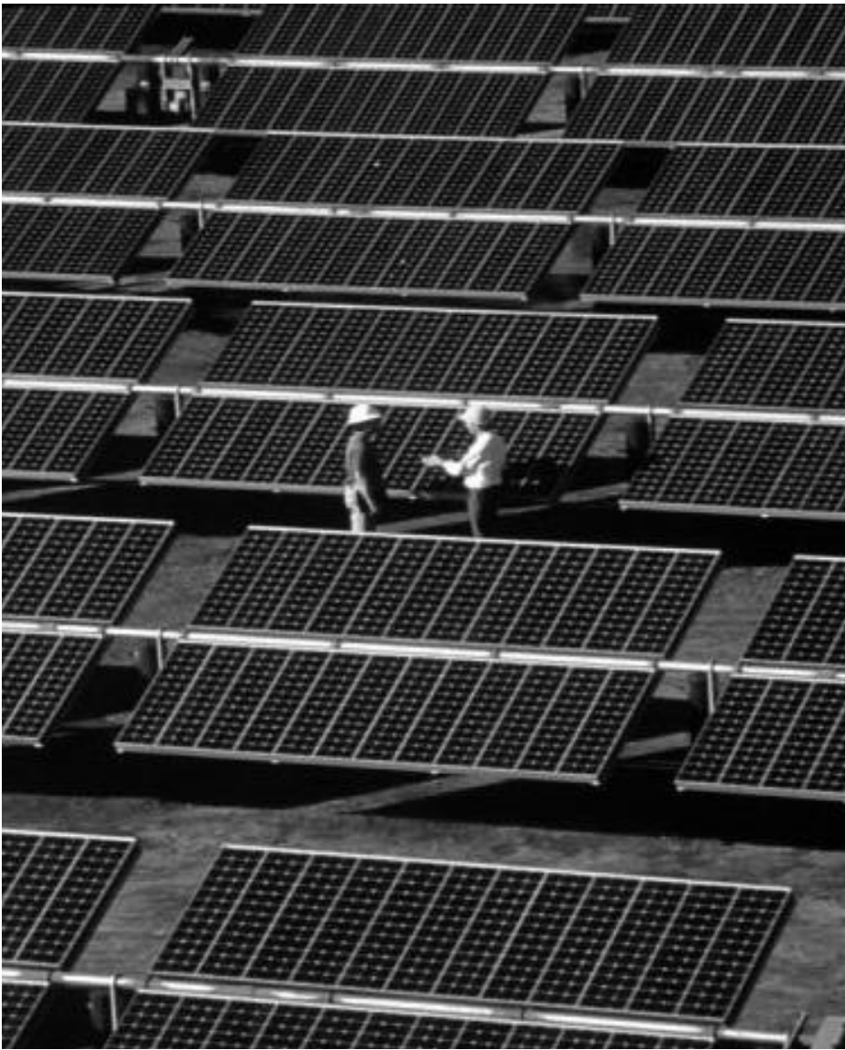
Crystalline silicon modules produced in the U.S. dominate the world market for PV. The Sacramento Municipal Utility District (SMUD) installed this 210-kilowatt crystalline silicon system at its Hedge substation in California.
