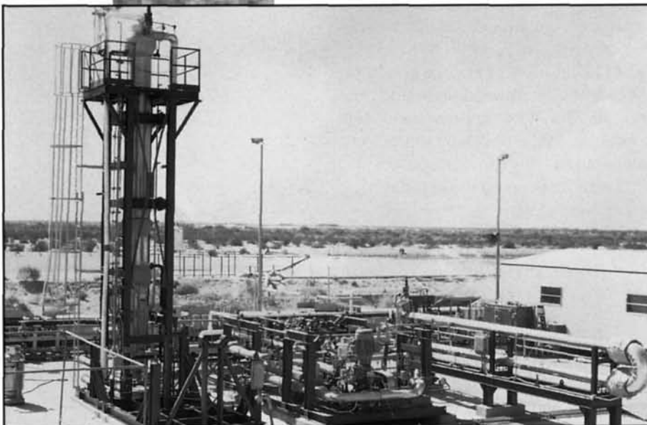
The Heat Cycle Research Facility (HCRF) has been used to evaluate advanced binary power systems in California's Imperial Valley since the mid-1980s. Techniques proven at the HCRF could boost binary power plant performance by 20%.
