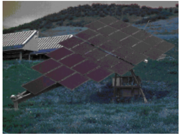
Fig. 4. APS 1.5 kW a-Si system
