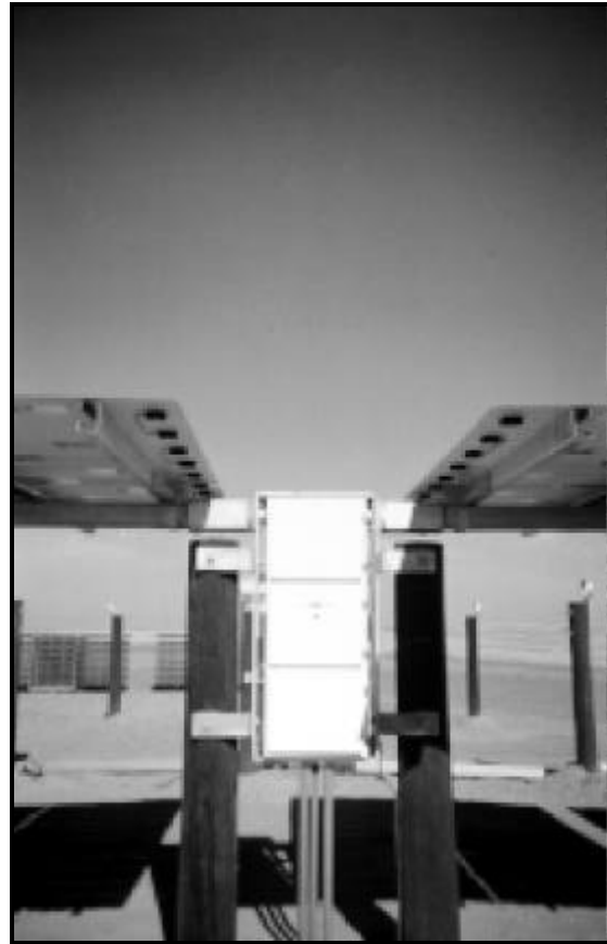
Figure 3: Photo by Utility Power Group, Inc. illustrating the Integrated Power Processing Unit and factory-assembled Modular Panels.
