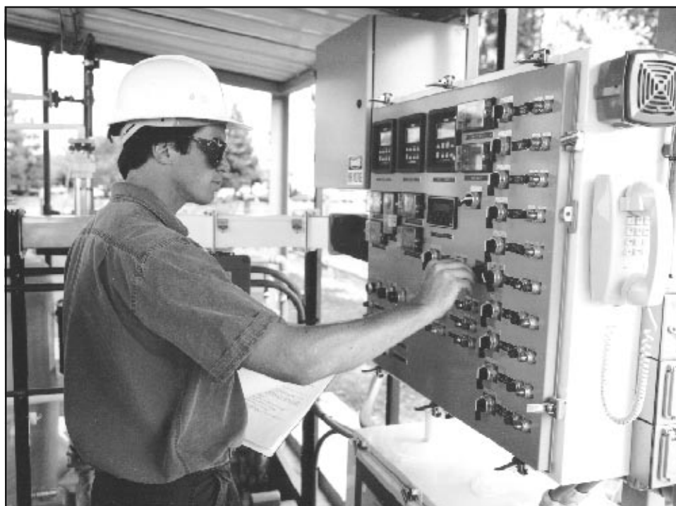
SI Program researcher monitors solar detoxification field test at a superfund site in California.
