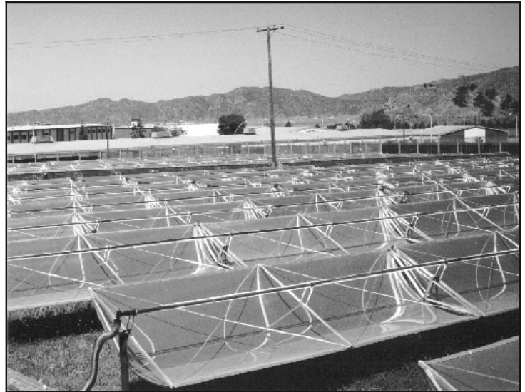
The solar collector field at the state prison in Tehachapi, California. This system heats water for the kitchen, bathing, and laundry facilities, supplying 7.2 billion Btus of thermal energy annually to the 5100-inmate prison. The system is part of the SI Program's Solar Process Heat Monitoring Project begun in 1994.
