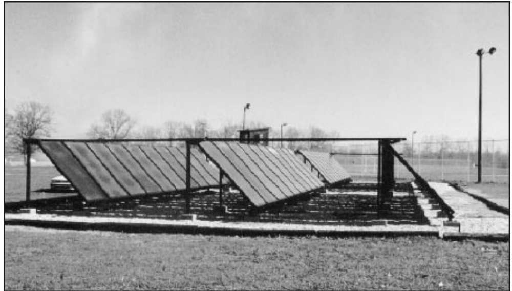
The flat-plate water heating system at the Caroline Correctional Facility outside of Richmond, Virginia. Installed in 1994 as part of the SI Program's work with state governments, the system supplies 30% of the hot water for the 140-inmate facility.
